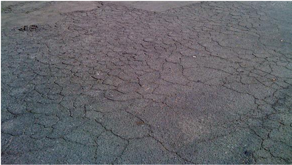
Fig. Alligator Cracking
