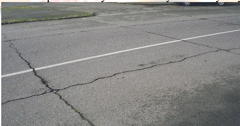
Fig. Joint Reflection Cracks
