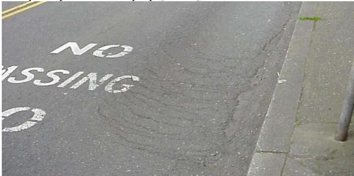
Fig. Slippage Cracks
