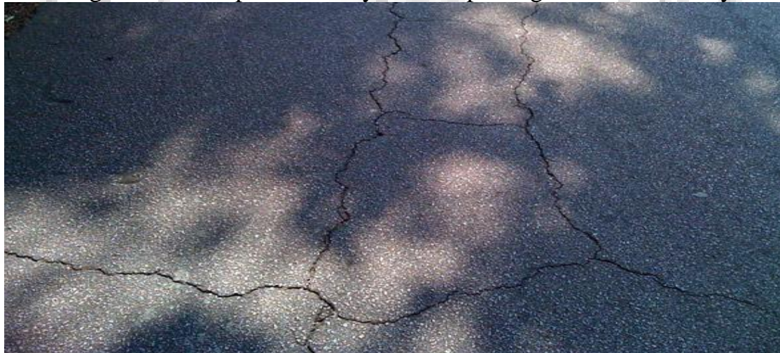
Fig. Block Cracking
