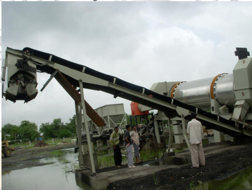
Fig. Load Out Conveyor
